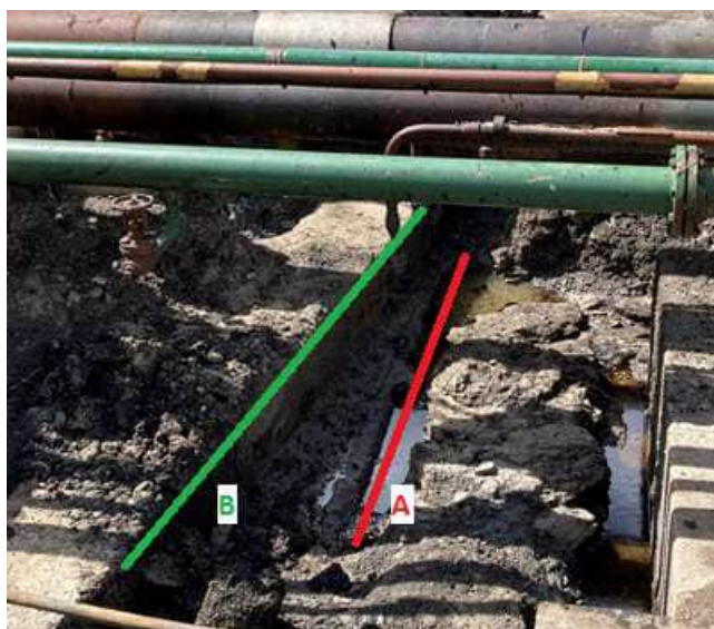
Figure B. Services Beneath the HFO Spill – Middle Trench
